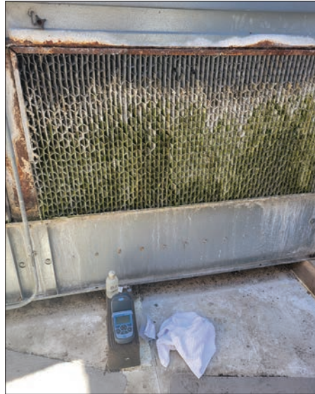
Photo 2. Staff from the Centers for Disease Control and Prevention (CDC) inspect a poorly maintained cooling tower during a Legionella outbreak investigation. Inadequately maintained cooling towers can aerosolize water containing Legionella bacteria. Photo courtesy of Nakia Clemmons, CDC.
